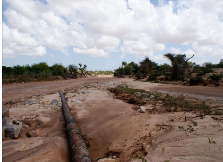
Existing pipeline (old and dilapidated)
